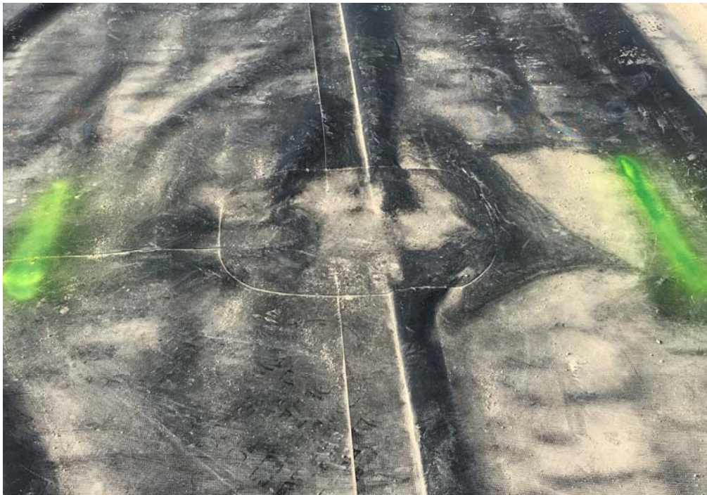
Photograph 8: Leistered patch needing extrusion welding in Contract A - Storage Lagoon.
