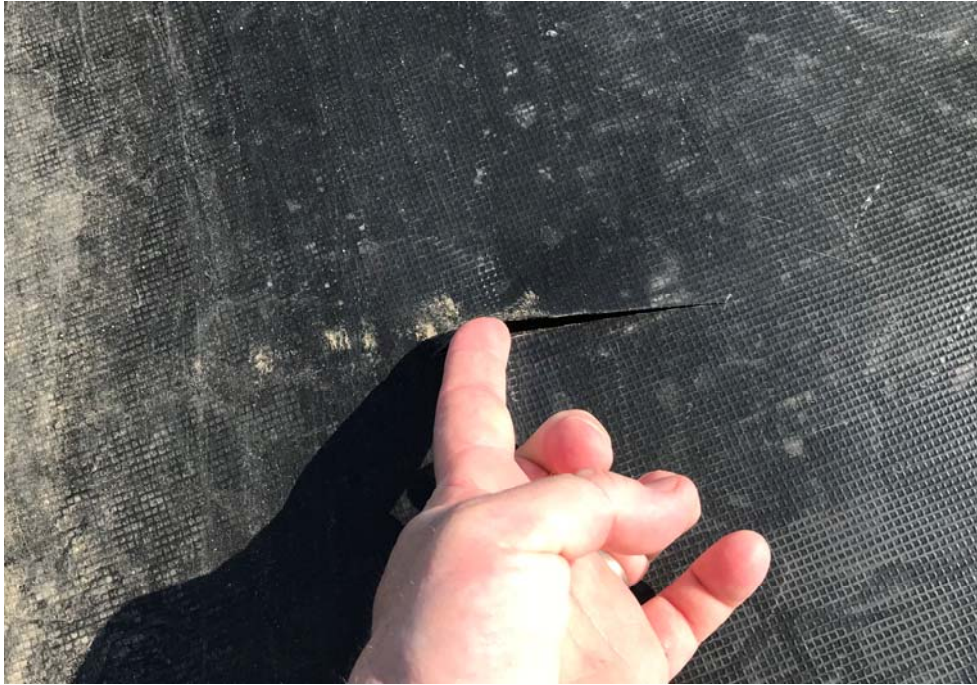
Photograph 5: Slice in the liner of the Contract A - Storage Lagoon.
