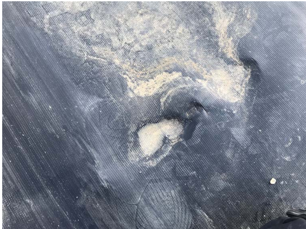
Photograph 6: Puncture in the liner of the Contract A - Storage Lagoon.
