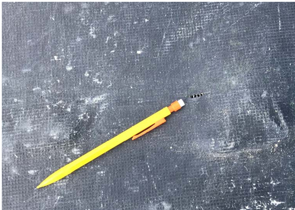
Photograph 4: Hole in the liner of the Contract A - Storage Lagoon.
