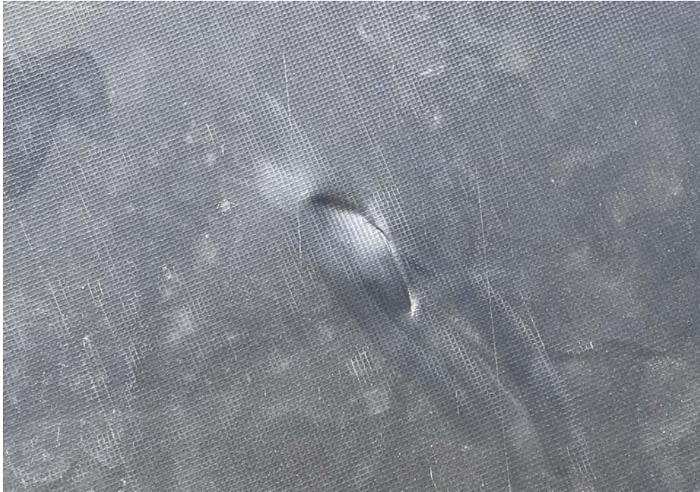
Photograph 7: Incursion in the liner of the Contract A - Storage Lagoon.
