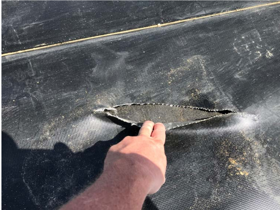
Photograph 3: Rip in the liner of the Contract A - Storage Lagoon.
